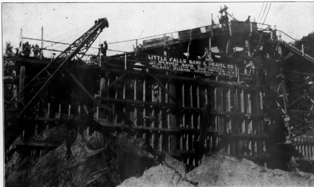
General View of the Plant. Little Falls
